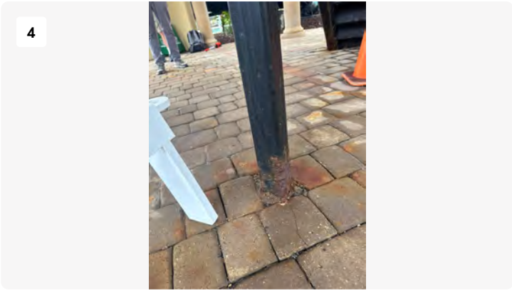
Corrosion at base:
