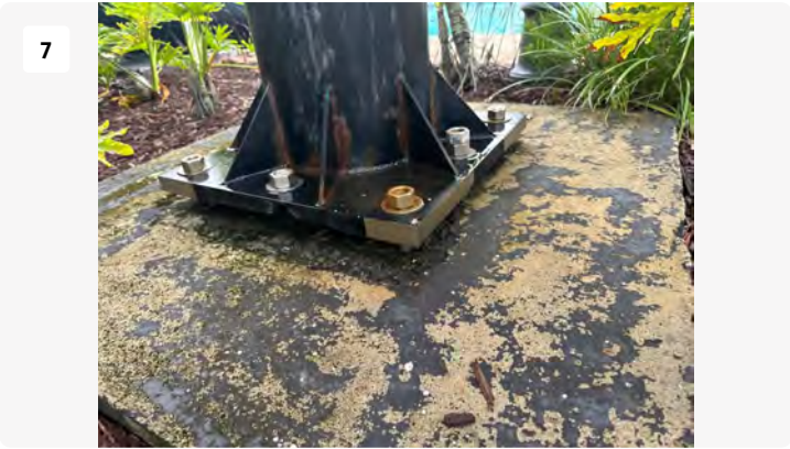
Some coating failure and surface rust on the welds:
