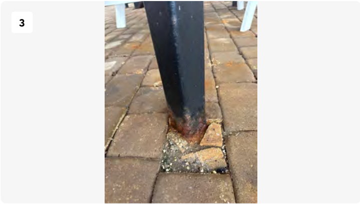
Corrosion at support base:
