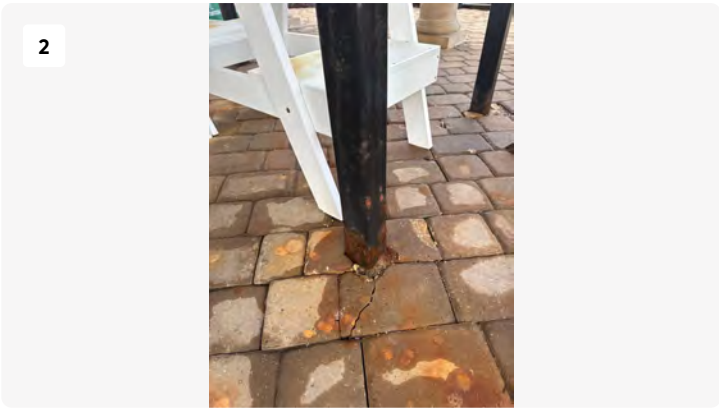
Corrosion at support base:
